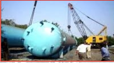
GFL Site A&H Plant Dahej
