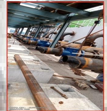
Meghmani Organics Ltd. Utility Piping
