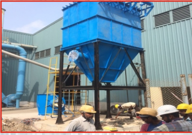
De-dusting Unit Project Rockwool Site Dahej
