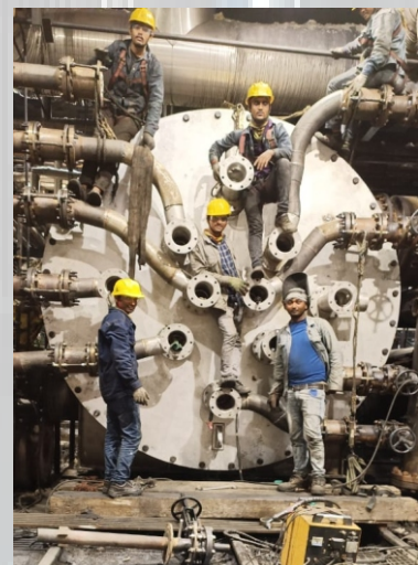
Epsilon Carbon Furnace Inconel Piping
