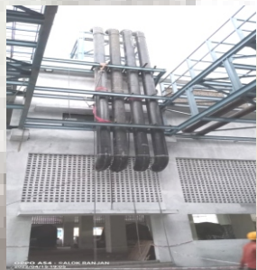
MEGHMANI ORGANICS UNIT-5 UTILITY PIPING
